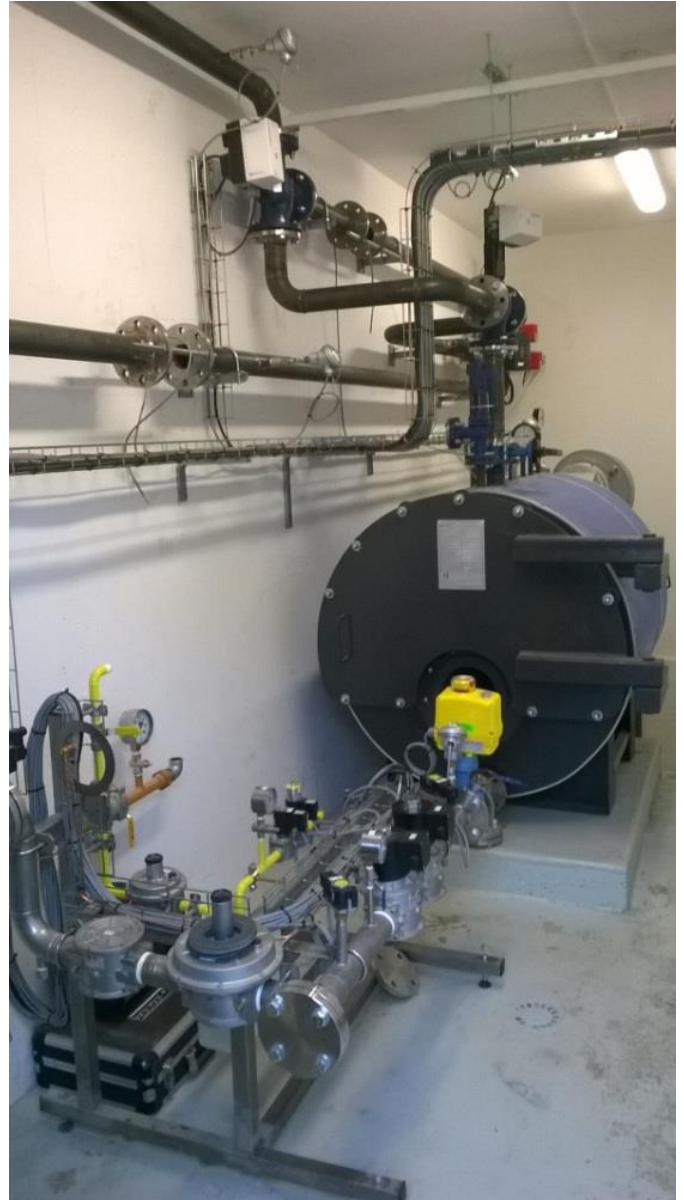
250 kW boiler for valorizing syngaz produced by a biomass gasification unit
