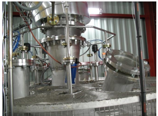
View of the upper side of a combustion chamber equipped with a VEGAR burner
